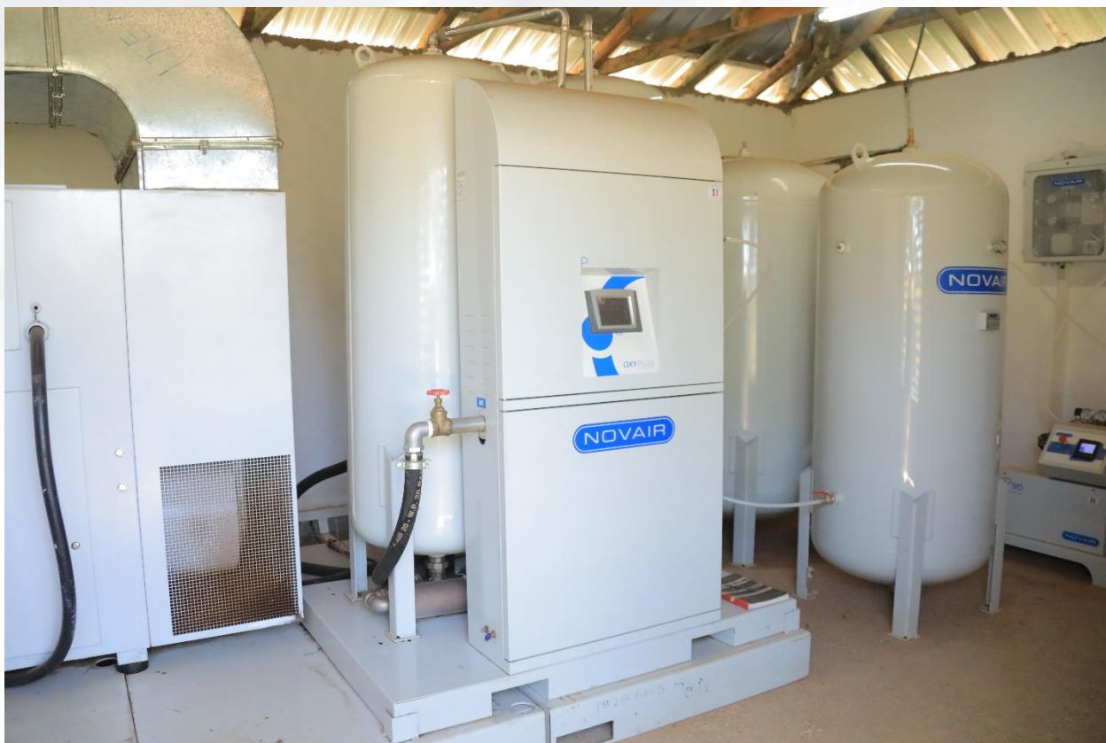
Figure 6. Oxygen Plant at Iten County Referral Hospital
