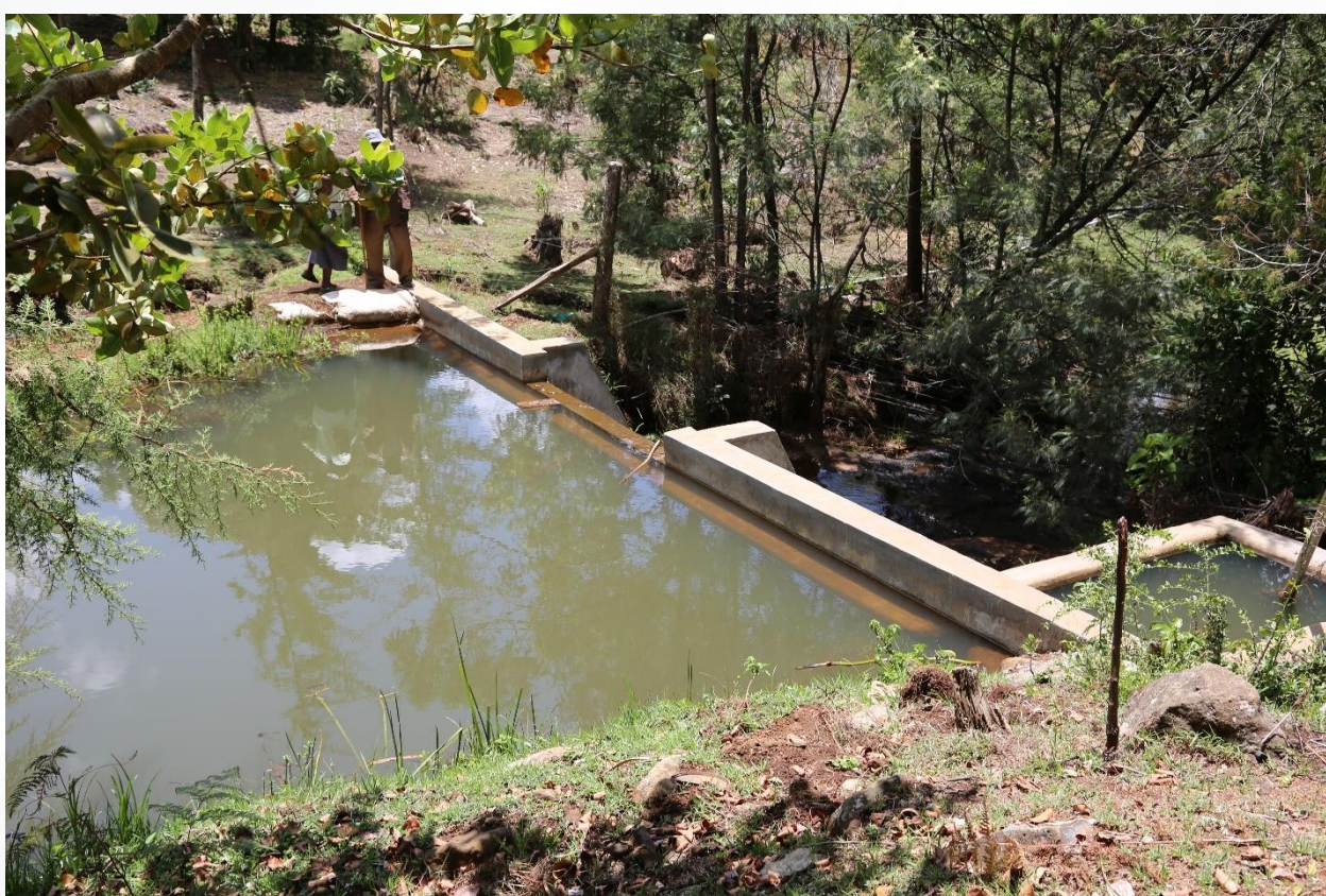
Figure 7. Chelut Water Intake
