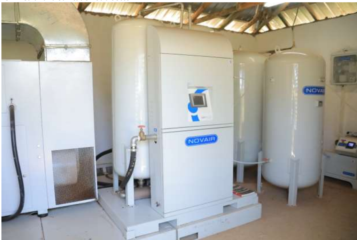
Figure 6. Oxygen Plant at Iten County Referral Hospital
